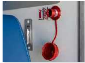
New receptacle in AFT cargo partition
